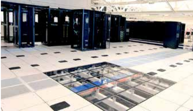
16,000 sq. ft. isolated floor system at UC Berkeley.
