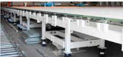
16,000 sq. ft. isolated floor system at UC Berkeley.
