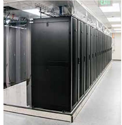
40' long Isolated Platform houses two banks of servers and IT equipment.
