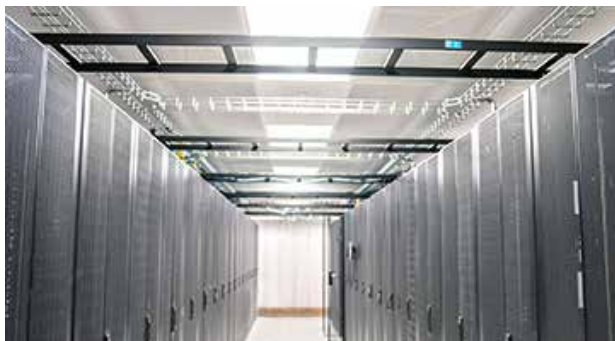
Overhead cable trays are easily used with DIS' Isolated Platform.
