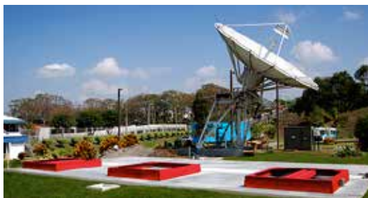
A modular isolation system ready to accept modular data center.
